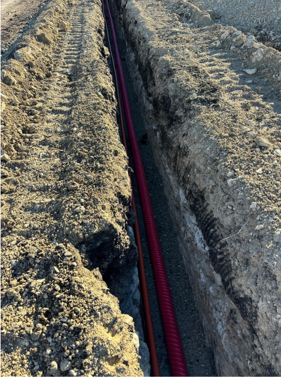
NextEra Solar project located near Gainesville, TX
